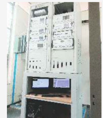
Rack-mounted PM, Gas Analyzers and Calibration Units inside the AAQMS
