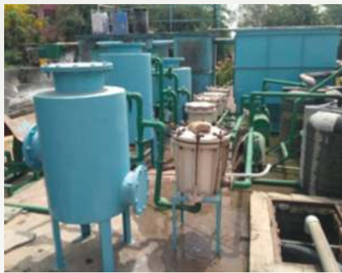
ETP Laundry Unit
