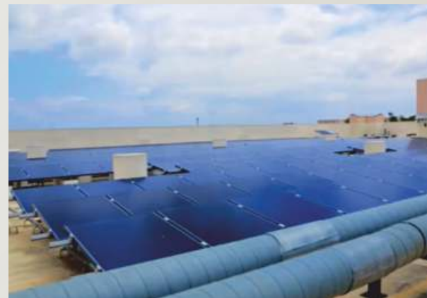
Rooftop Solar PV plant
